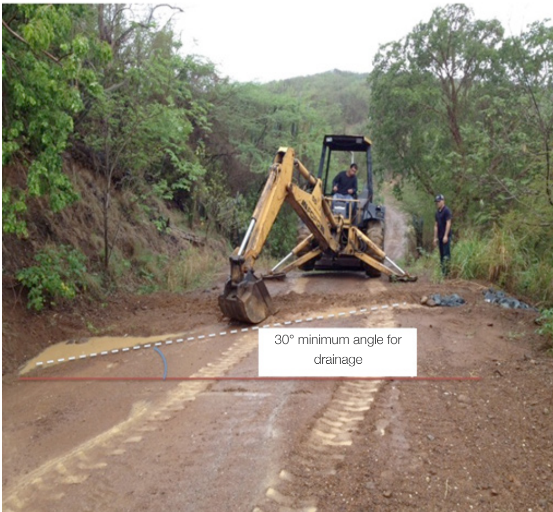
Figure 3. Example of a concrete or earthen water bar under construction (based on NYSF, 2011)
